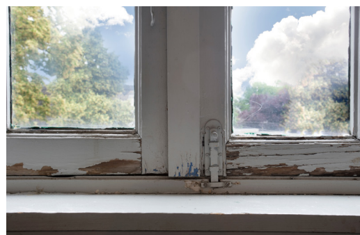
4 Flaking paint on wooden sg windows
