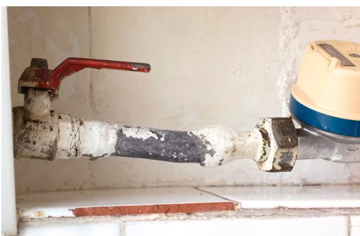
2 Original lead pipe at stoptap
